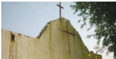
This church near Sharakpur was damaged in a confrontation between Christians and Muslims in August. Through the Fellowship of Christ we will provide funds to repair the church.
